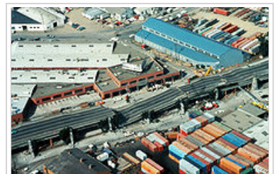
Portion of the collapsed Cypress Viaduct in Oakland.
