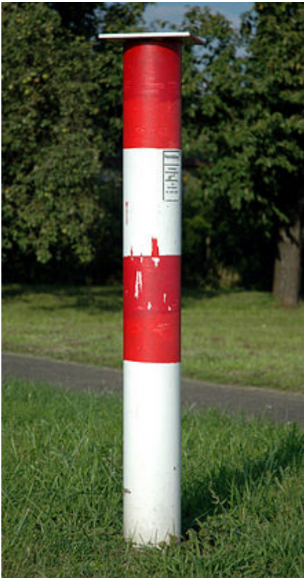
CEPS pipeline marker near Untergruppenbach in Germany
