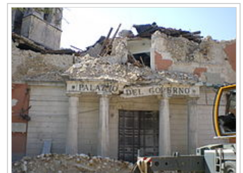
The local prefecture (a government office) damaged by the earthquake.
